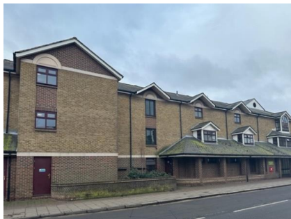
Urban design: These schemes both present poor frontages with poor doors windows and shopfronts. These schemes present a poor urban design. The character of the Conservation Area is based on active frontages, with
